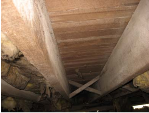
Lack of under floor insulation
