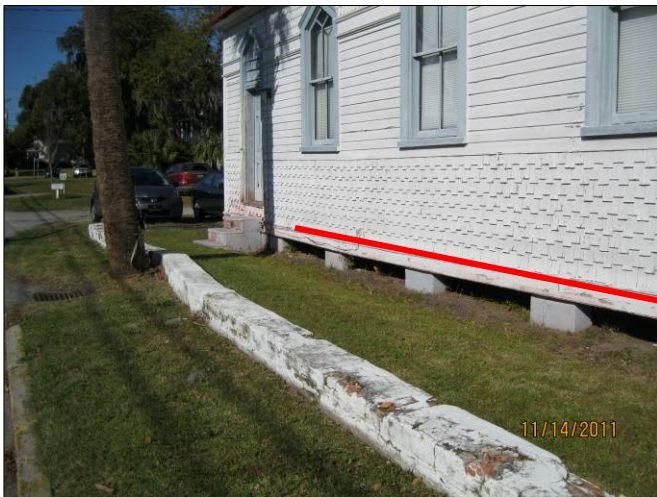
S-5 Left side appears to be sagging slightly
