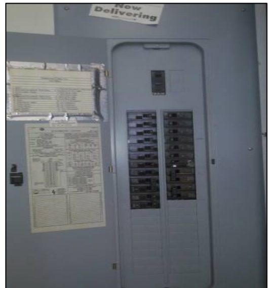
E-2 Electric Panel
