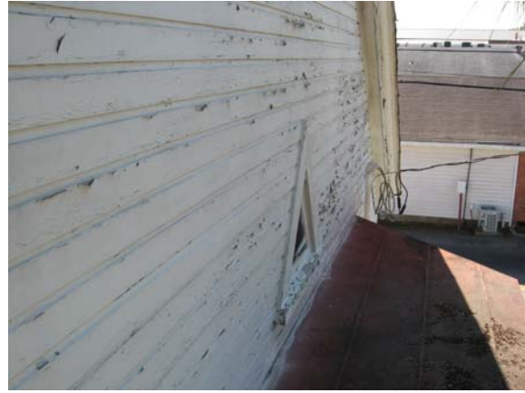
Peeling paint at rear gable
