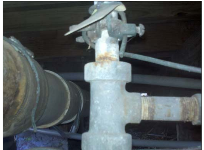
P-2 Water Riser
