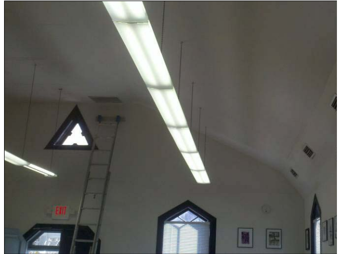
HVAC -4 Sidewall Diffusers
