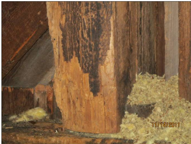
S-1 Vertical post with insect damage
