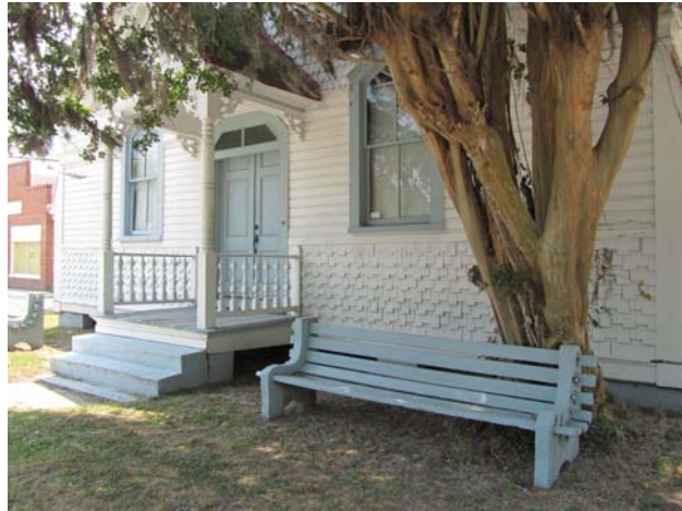
Irregular risers at front entry steps
