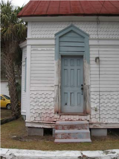
Deteriorated south rear door
