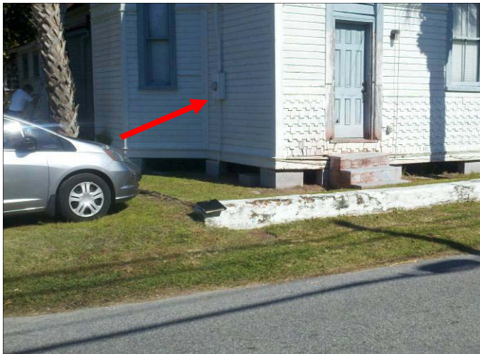
E-1 Electric Meter
