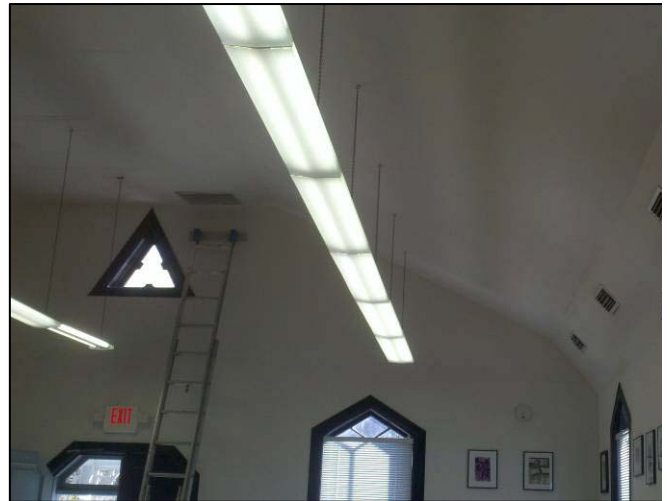
E-4 Overhead lights
