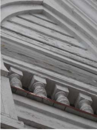
Peeling paint at Belfry
