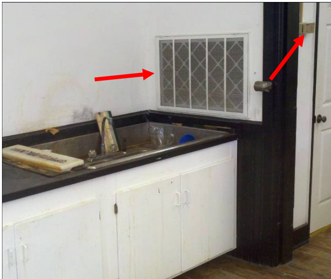
HVAC -5 Thermostat and return air grill
