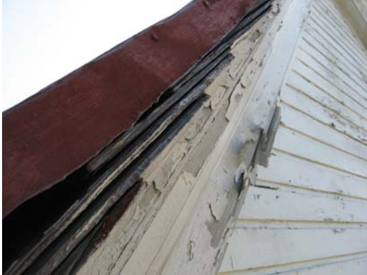
Wood shingles exposed under metal roof
