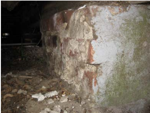
Deteriorating mortar at support wall
