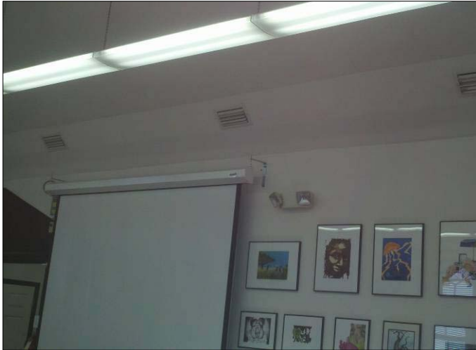
HVAC -3 Sidewall Diffusers
