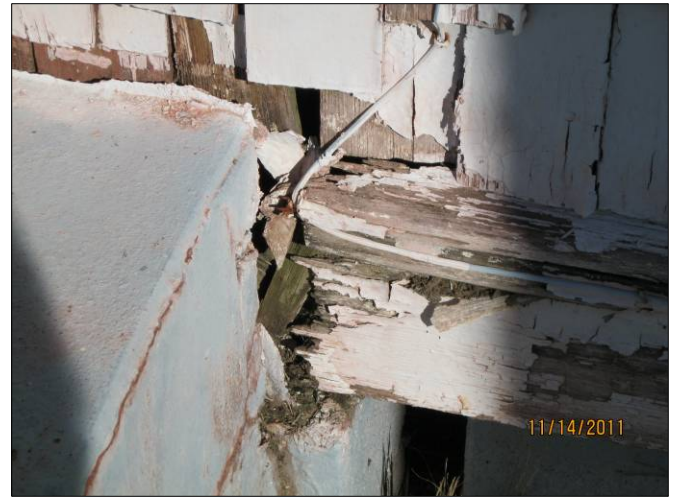
S-4 Deteriorated wood at right side of door
