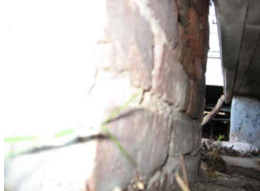
Deteriorated chimney base mortar
