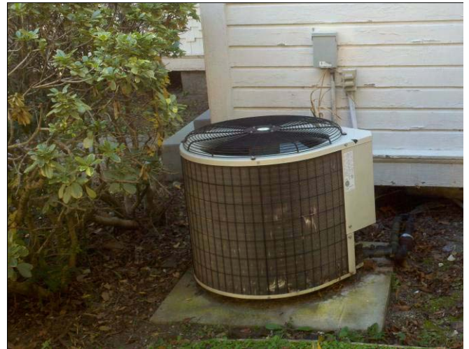
HVAC -2 Condenser unit
