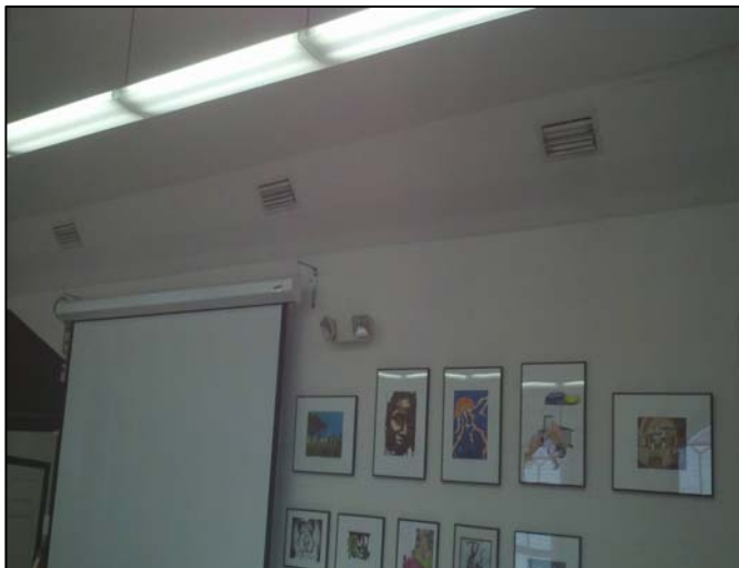
E-7 Emergency lights
