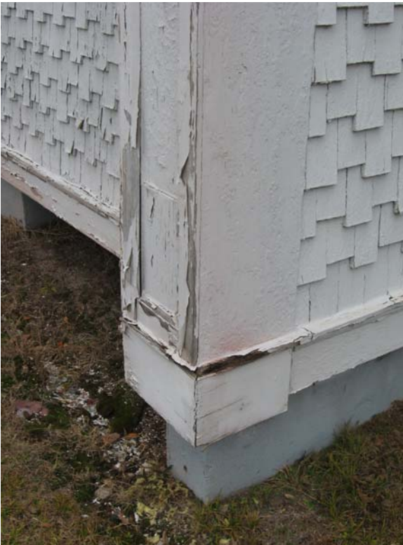
Peeled paint chips at ground
