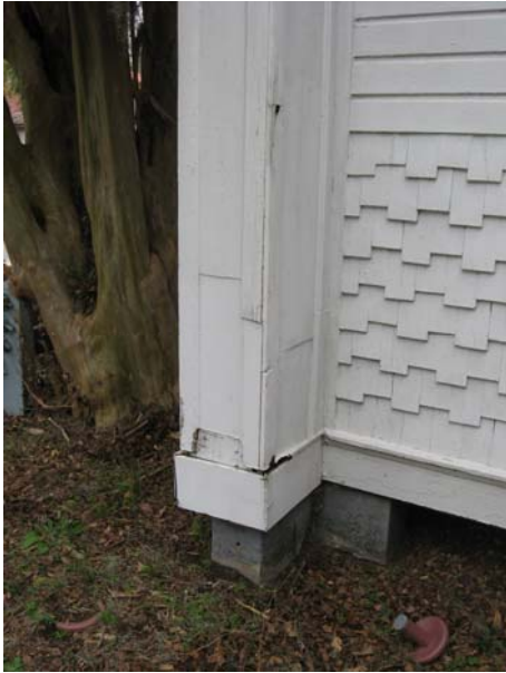
Mismatched wood patch
